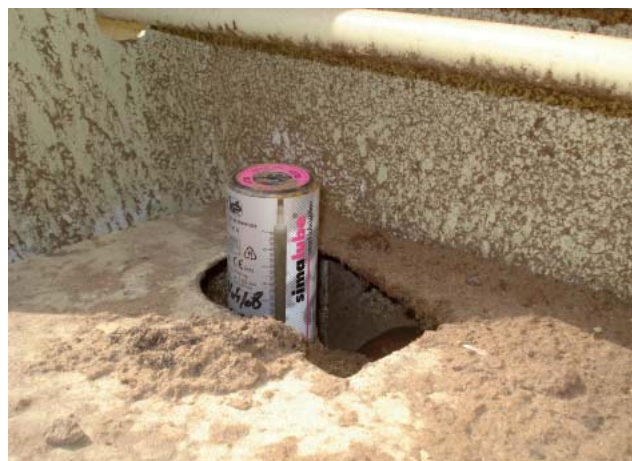
Difficult to access lubrication points
