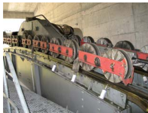
simalube ® is used to lubricate the carrying cable of the Matterhorn Glacier Paradise cable car.
