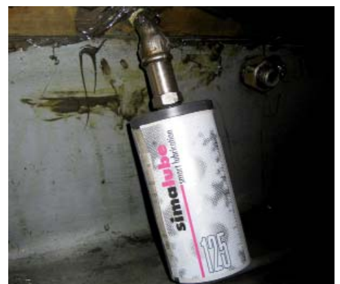
Detailed picture of the lubrication of a carrying cable.
