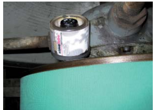
Lubricating the bearings on the drive shaft of a belt with a 30ml dispenser.
