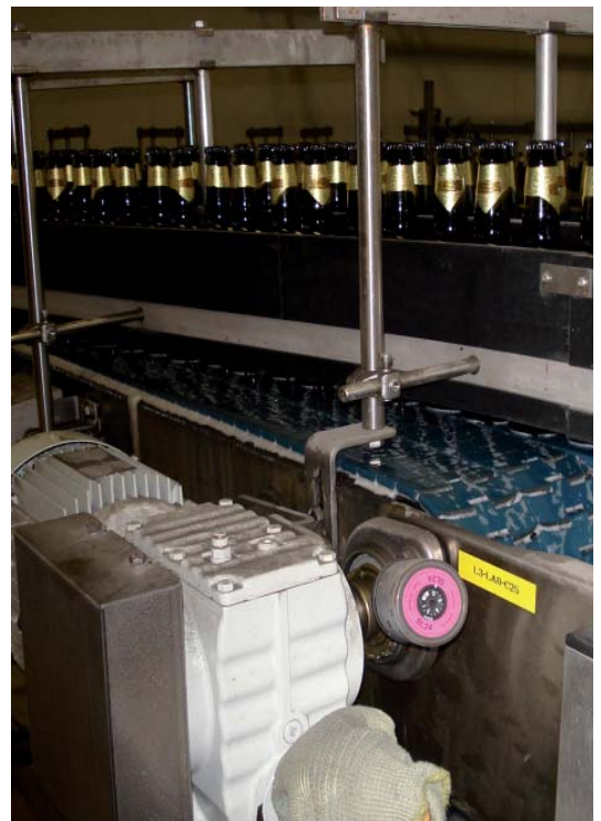
Reliable greasing of a driving shaft with simalube ®.
